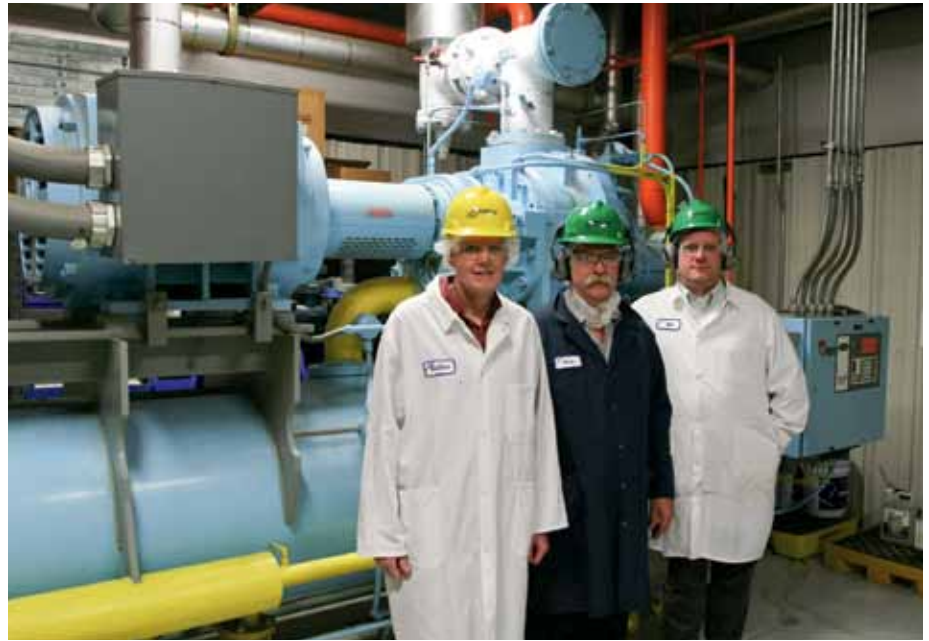
From left: Pacific Power's Chuck Phinney, J&J Snack Foods plant engineer Brian Stoddard and plant manager Rob Tiberino get a look at the plant's energy-saving upgrades installed with help from Energy Trust of Oregon.
